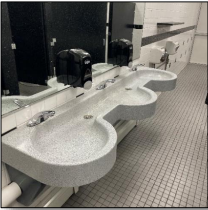
Newer sinks and fixtures with touch control in restrooms
