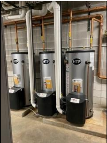
Three domestic HW Heaters in good condition
