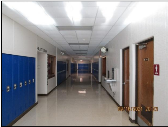
Corridors with CMU, corkboard, VCT and ACT are in good condition and well maintained
