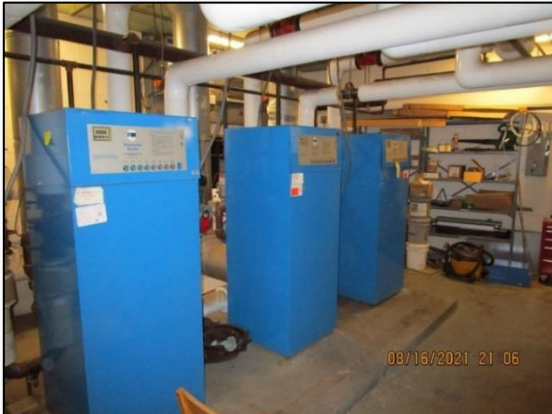
Three of the five Patterson-Kelly gas-fired 2,000,000 MMbtu hot water boilers circa 1998 are in good condition
