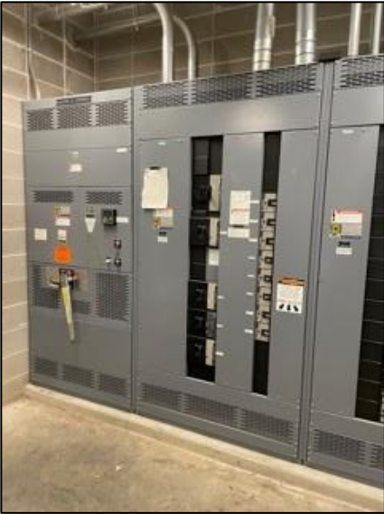
Building has a 3000 amp Main Distribution Panel, providing 480/277V to building
