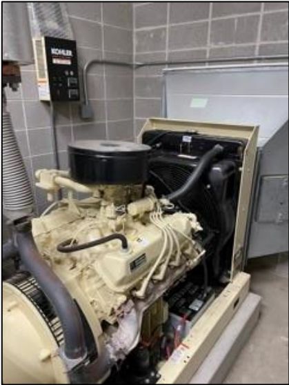
Building has an 80 kW generator in excellent condition
