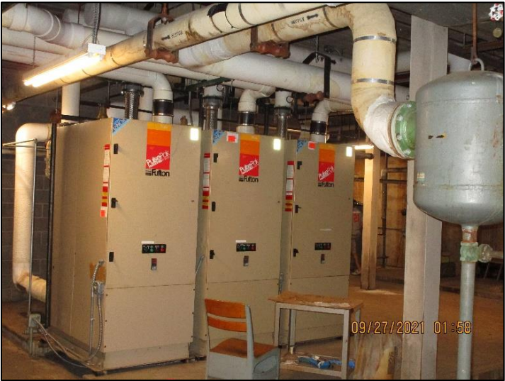
Three Fulton Boilers installed in 2004 are in good condition
