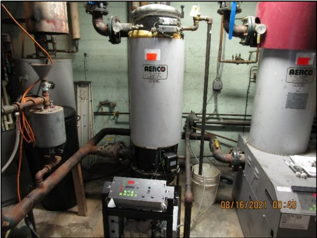
(1 of 2) Aerco hot water boilers are in good condition and well maintained. This one was in the process of being rebuilt
