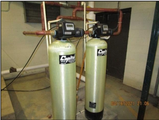
Duplex water softener installed in 2018 for boiler and domestic water
