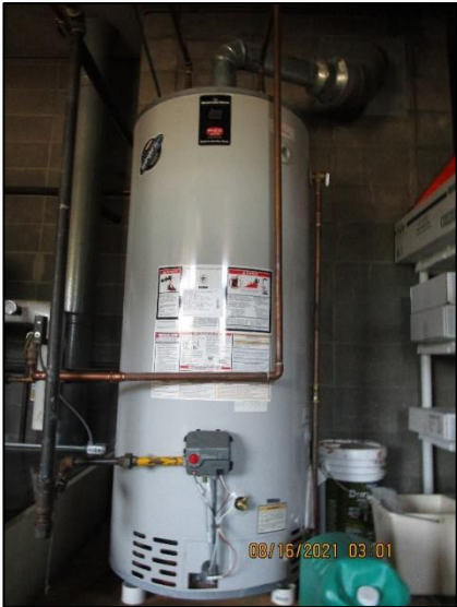
New energy saving water domestic hot water heater installed
