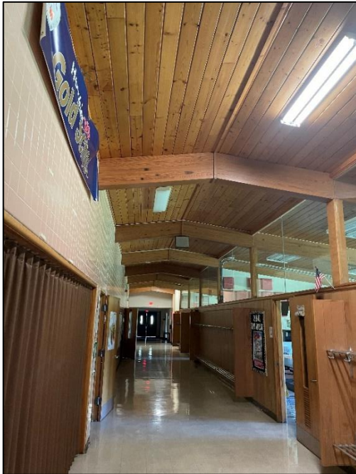
12" x 12" VCT on floors in corridors and classroom. 1 ¼" tongue and groove wood ceiling are in good condition
