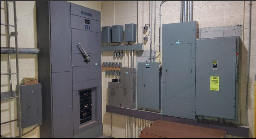
The existing aged incoming electrical main incoming switch and distribution panels behind gymnasium.
