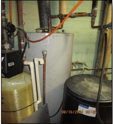
80-gallon gas-fired domestic hot water heater and water softener installed in 2018 in good condition
