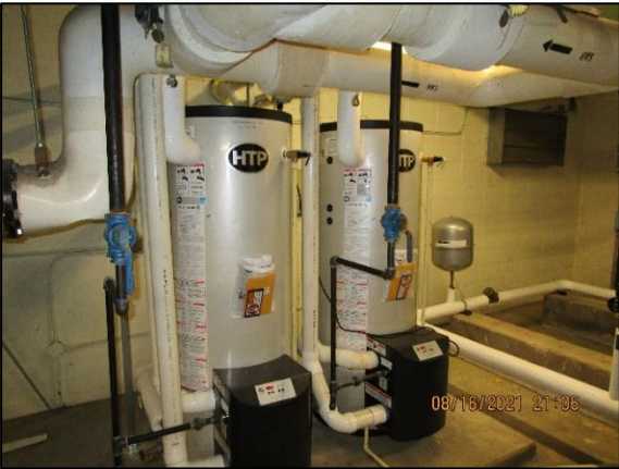
Brand new two 120-gallon gas-fired domestic hot water heaters installed February 2021
