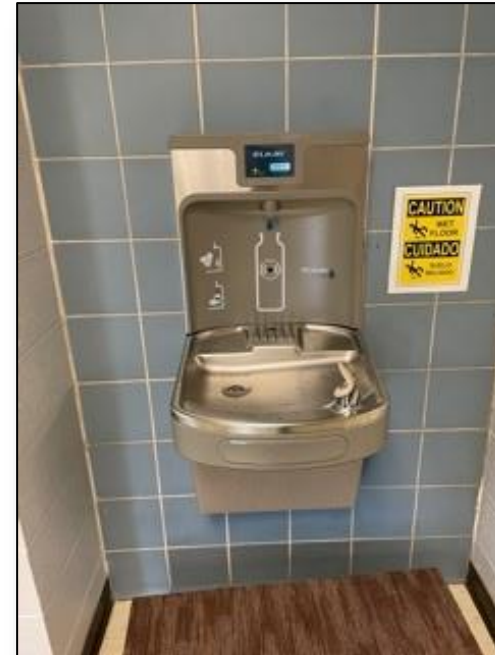
New energy efficient water fountains installed
