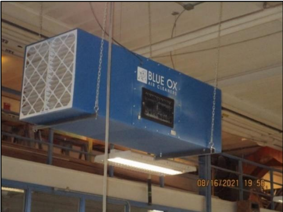
Wood Shop has 3 air scrubbers for dust control
