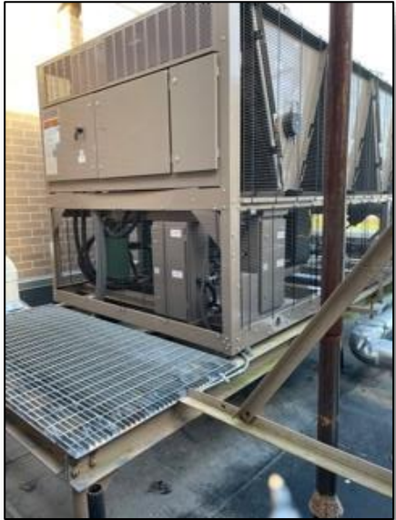
Building has 2 chillers installed in 2019 providing 250 tons of cooling throughout building
