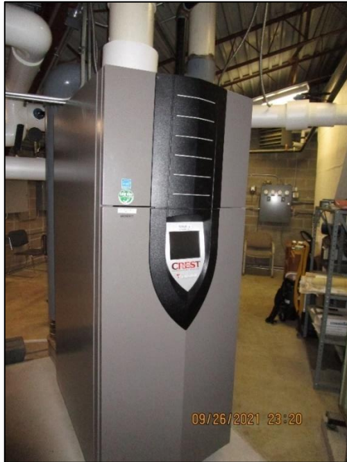
Newer Lochnivar boilers installed in 2018 are in good condition
