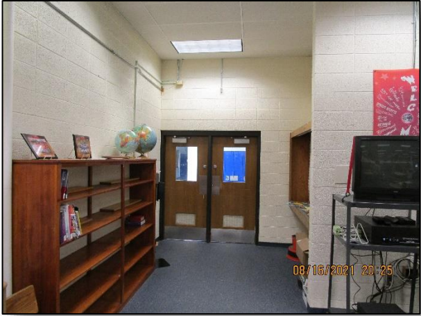
Library and other rooms limited egress and exit signage which would cause confusing during an emergency evacuation.
