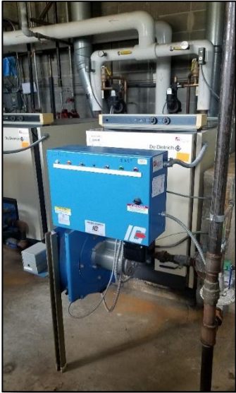
Boilers are in good condition and well maintained
