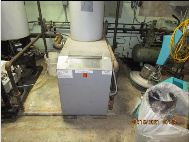
(2 of 2) Aerco hot water boilers are in good condition and well maintained.
